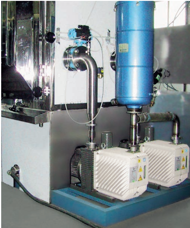
Freeze Drying equipment.
